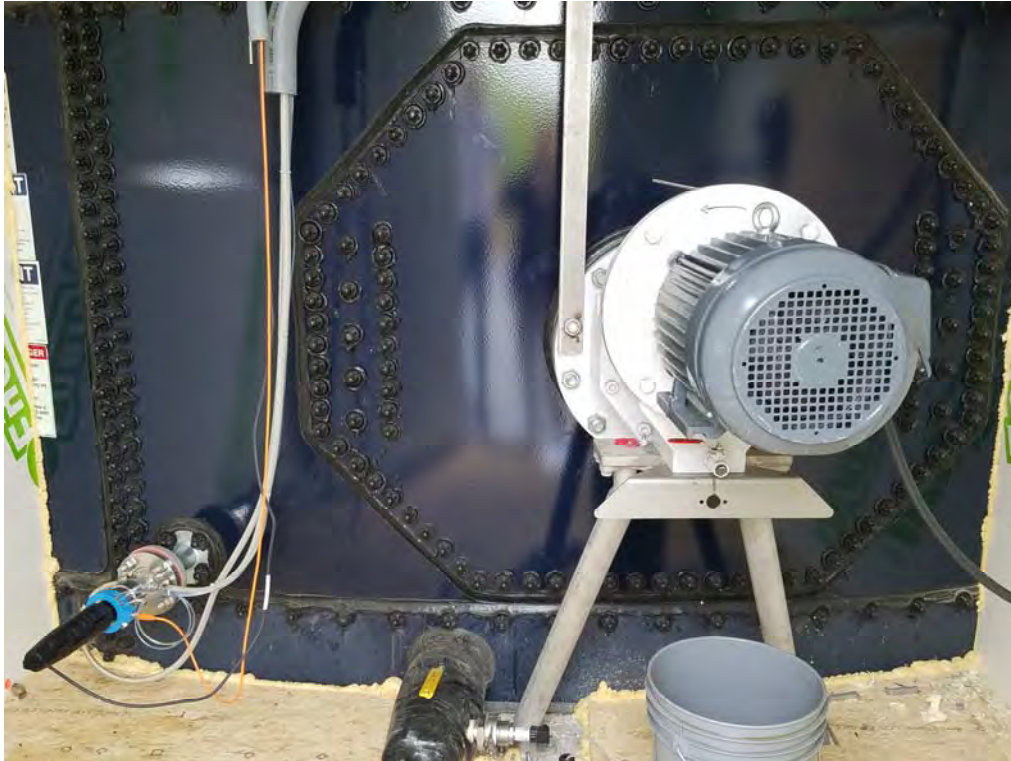
Storage Tank 1: pH probe and Agitator, photo taken by Kim Watson, 5/22/2018
